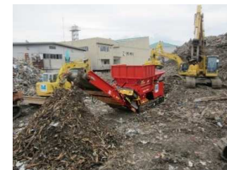
Separate process of large quantities of garbage generated by the Tohoku Earthquake using wood crushers
