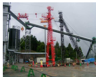
Cable cranes play an active role in transporting materials during construction of dams and power plants
